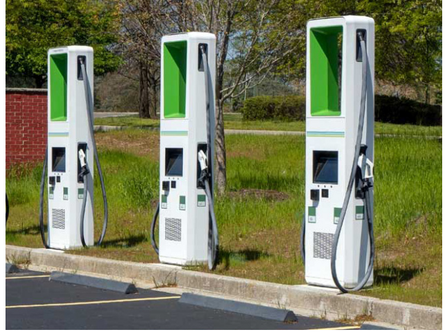
Electric Charging Station
