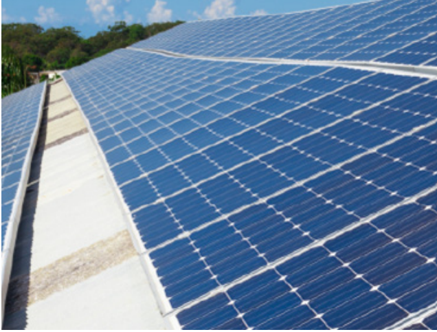
Photovoltaic Solar Panels
