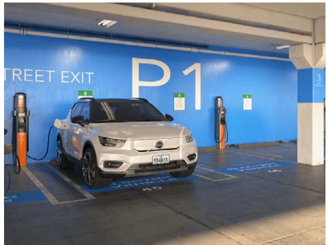
Electric Charging Station in Parking Structure
